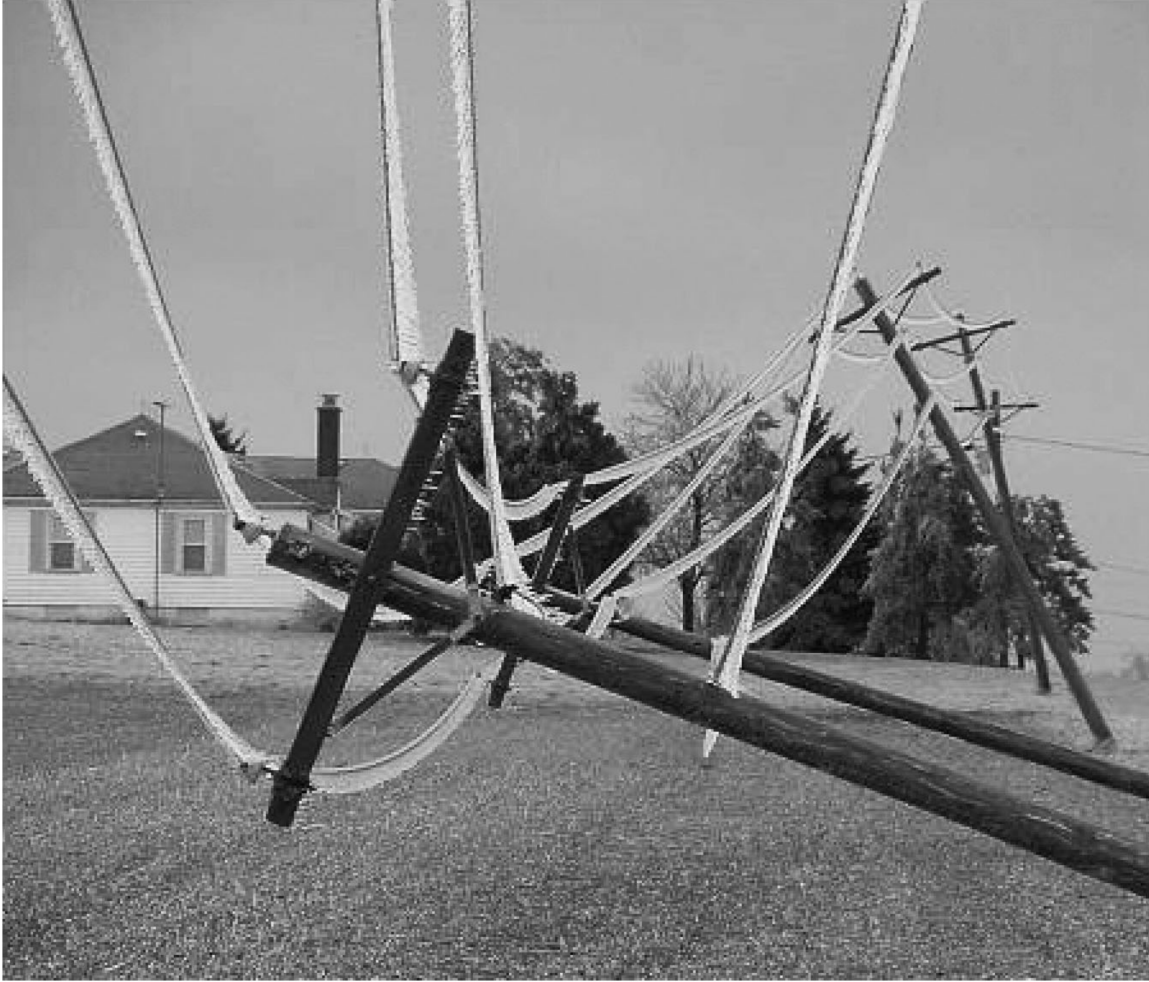
Figure 1. Image of fallen wood poles due to ice deposited on metal cables.
